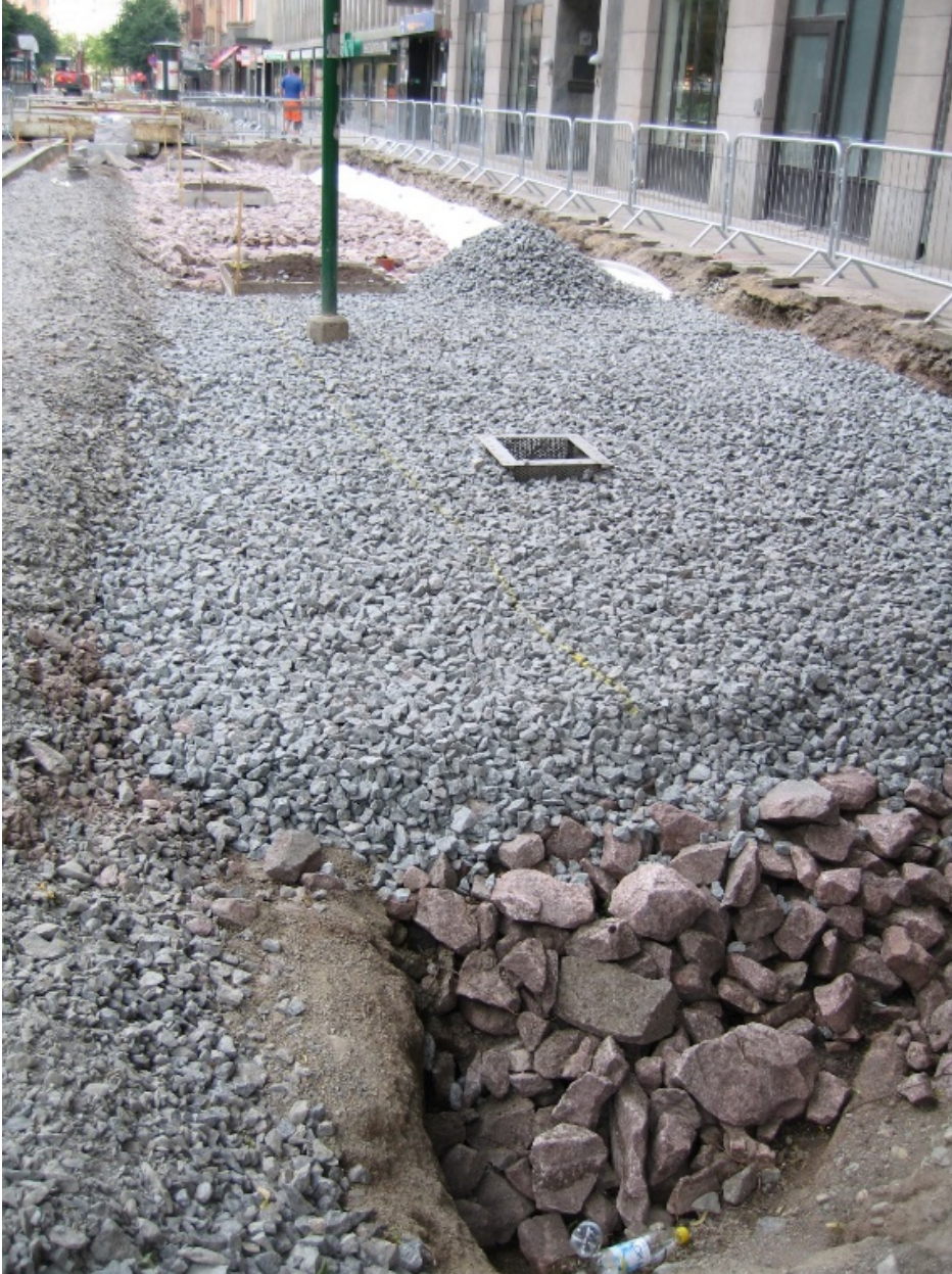
Figure 2- Stockholm Structural soil. This image shows a picture with the 100-150 mm skeletal soil on the bottom of a planting-bed. It has been topped by the 32-63 mm aerated bearing layer and the storm water inlets have been installed. Photo: Björn Embrén. Permission to publish has been granted by Björn Embrén.
