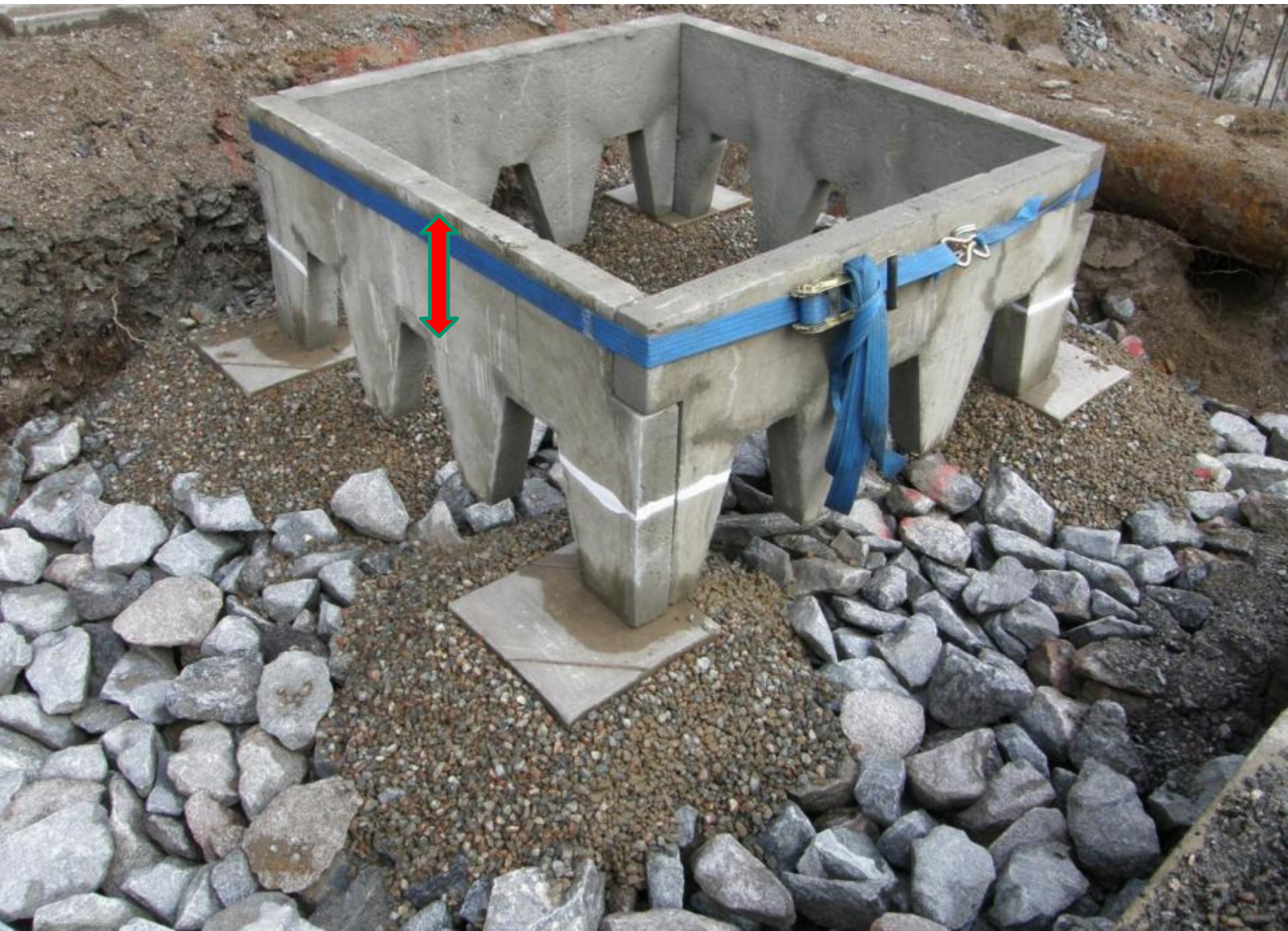
Closed top of the concrete box to hold the pavement and bearing layer in place
