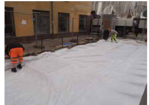
Geotextile extends across the leveling layer and the entire plant bed. It is important that the geotextile folds against tree-pit foundations, wells and edge supports to prevent the pavement bearing layer from being mixed with aerated bearing layer.
