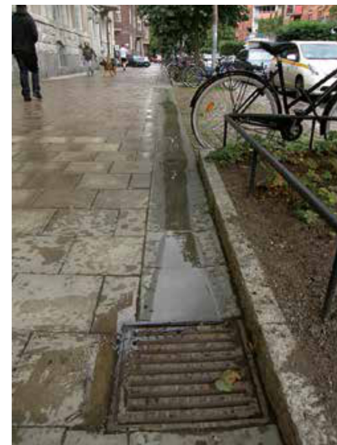
Rainwater drain with aeration well connected to plant bed.
