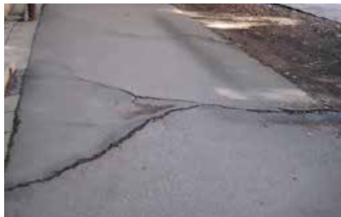
Damage to city surfaces caused by roots.
