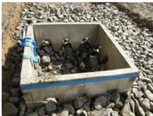
Stones that fall into the foundation openings mean that the foundation is fixed.
