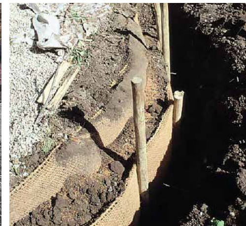
Root drapery of coconut carpet mounted on wooden stakes with moist soil. When backfilling cannot be carried out immediately, the root canopy protects the tree roots from dehydration.
