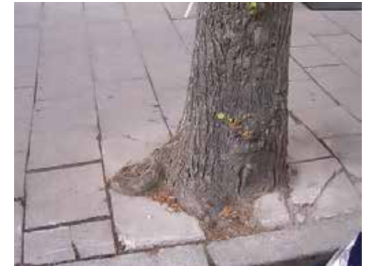
Pavement leaves no space for the tree trunk.
