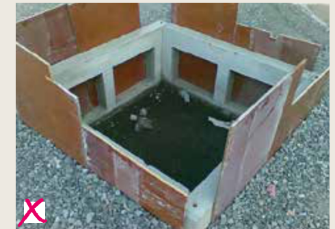
Incorrect design: boards have been set to prevent the structural soil from falling into the foundation. When the boards in the future collapse, the ground around the box will settle.
