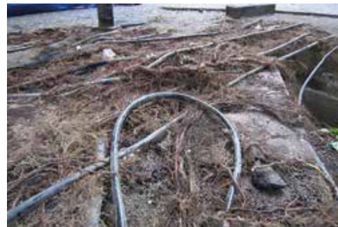
Roots and cables compete for space underground.
