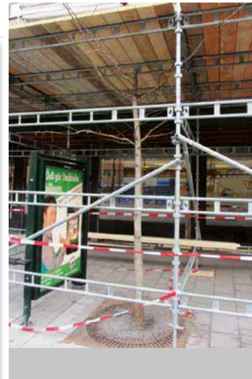
Example of damage: the tree has been sawn when mounting the scaffolding.
