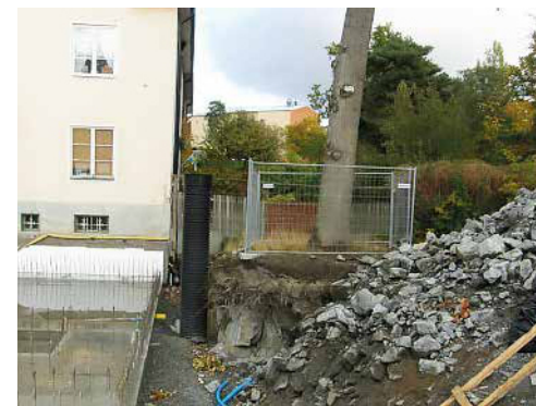
Not all trees can be saved during new construction. This tree has no chance of survival.
