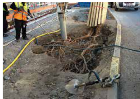
Vacuum excavation / exposure of root systems on adult trees with compressed air lance.
